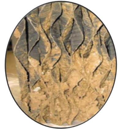
Fine particles clog the tower packing reducing the ability to cool the recirculation water.
